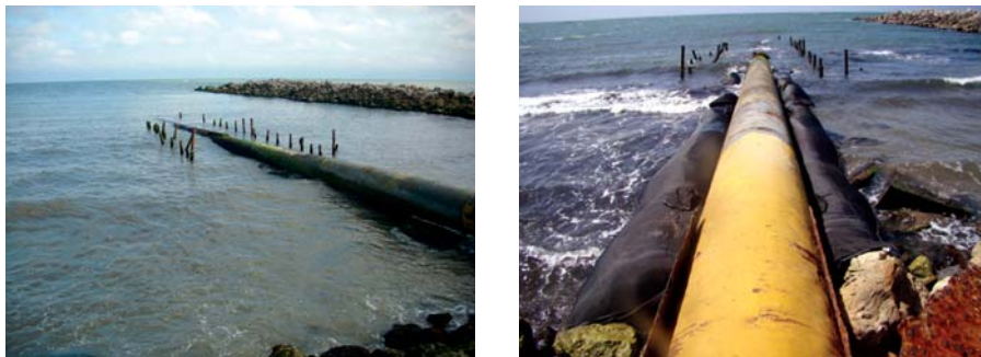
FIGURE 8 Before-and-after comparison for pipe 3
